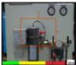
NEAR A IMPORTANT LEAK
