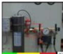
FACE A IMPORTANT LEAK
