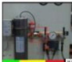
FACE A IMPORTANT LEAK
